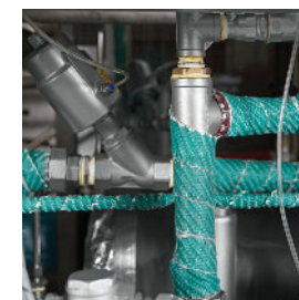
AISI 304 Stainless Steel Piping with Heat Insulation
